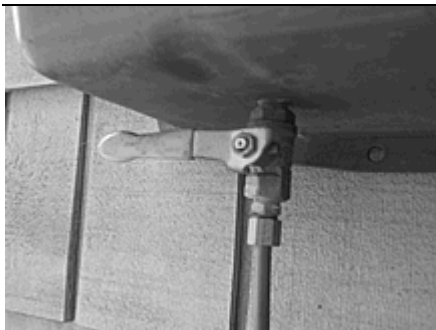
Tank Shut Off Valve
